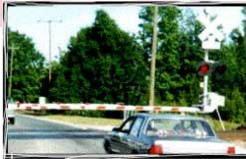
A Long Arm Gate extends over 3/4 of the roadway.
